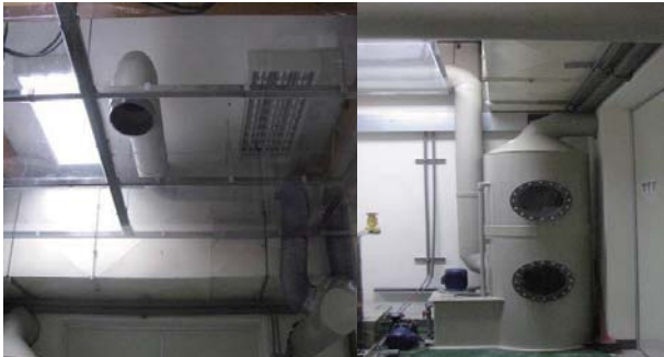
Fig. 4. Exhaust pipe and wastewater processing station.
