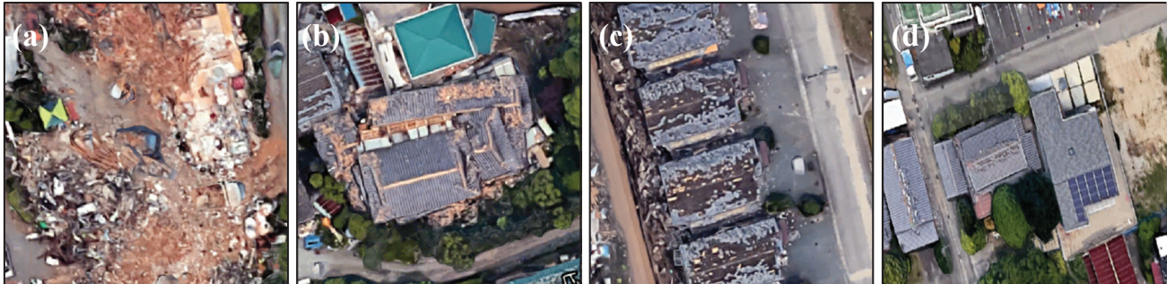
Fig. 2. Typical building damage patterns in the 2016 Kumamoto earthquake: (a) the buildings become debris; (b) the structure of buildings is severely damaged; (c) the roof tiles are severely damaged; (d) no significant damage can be observed.
