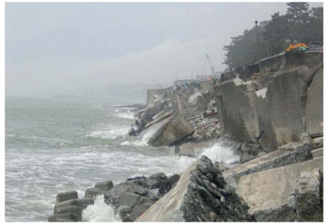
Fig. 4. Collapsed Seisho Bypass seawall, September 9, 2007.
