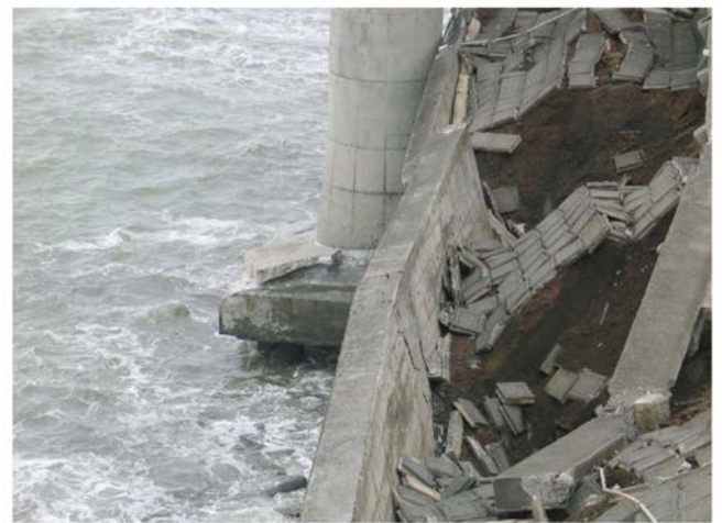
Fig. 5. Damaged Ginpa Bridge footing and tilted seawall, September 9, 2007.
