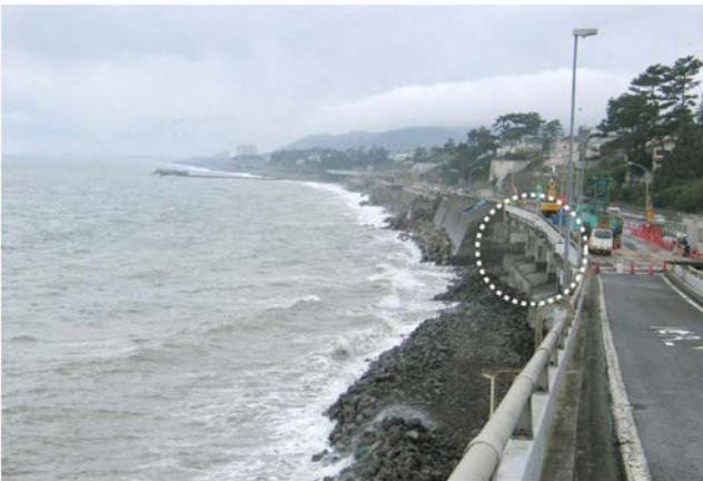
Fig. 8. Damaged Seisho Bypass seen from the top of the Ginpa Bridge looking west, October 8, 2007.
