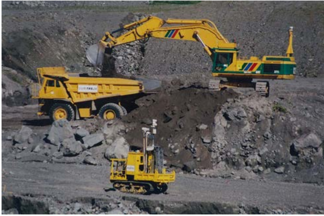
Fig. 9. Unmanned construction machinery developed ahead of the world and implemented for disaster prevention.
