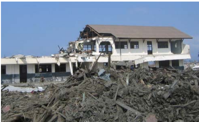
Fig. 3. Damage to Banda Aceh Junior High School No.5 building.
